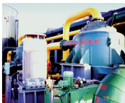
250t/h HiGee installation for seawater deoxygenation in offshore platform (Courtesy of Research Center of the Ministry of Education for High Gravity Engineering & Technology, University of Beijing)
